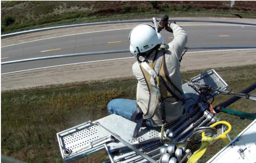
Working from a platform attached to a helicopter, a utility lineman attaches a spacer between transmission conductor.
