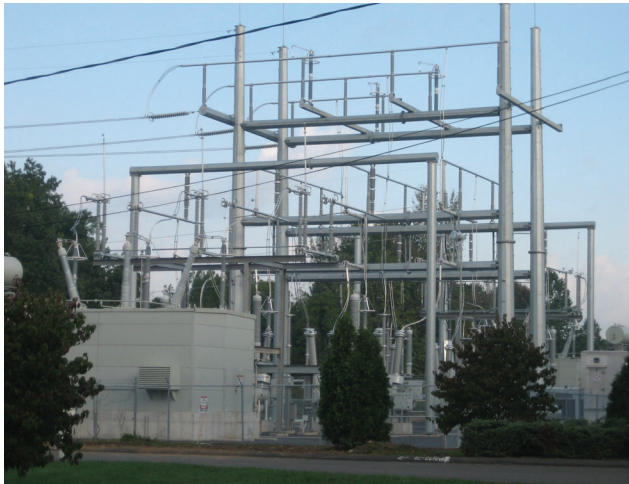
At either end of an underground section of the line, large one-acre transition structures (mini-substations) need to be constructed.
