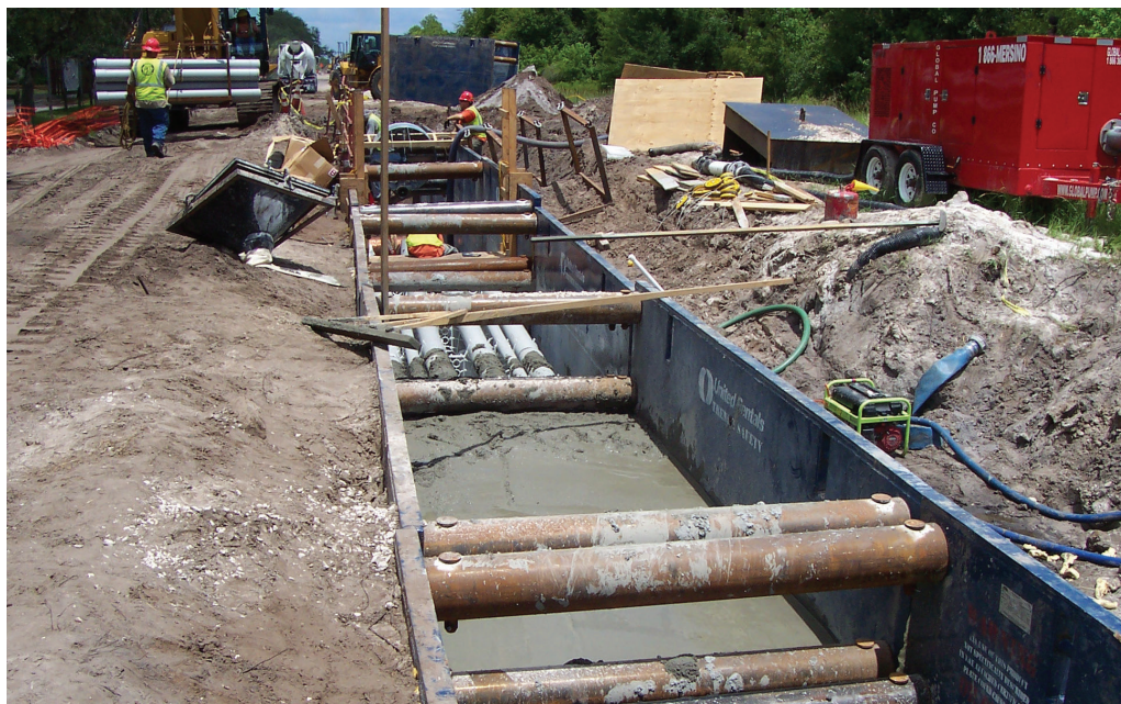
Transmission lines are installed in concrete-encased duct banks.
