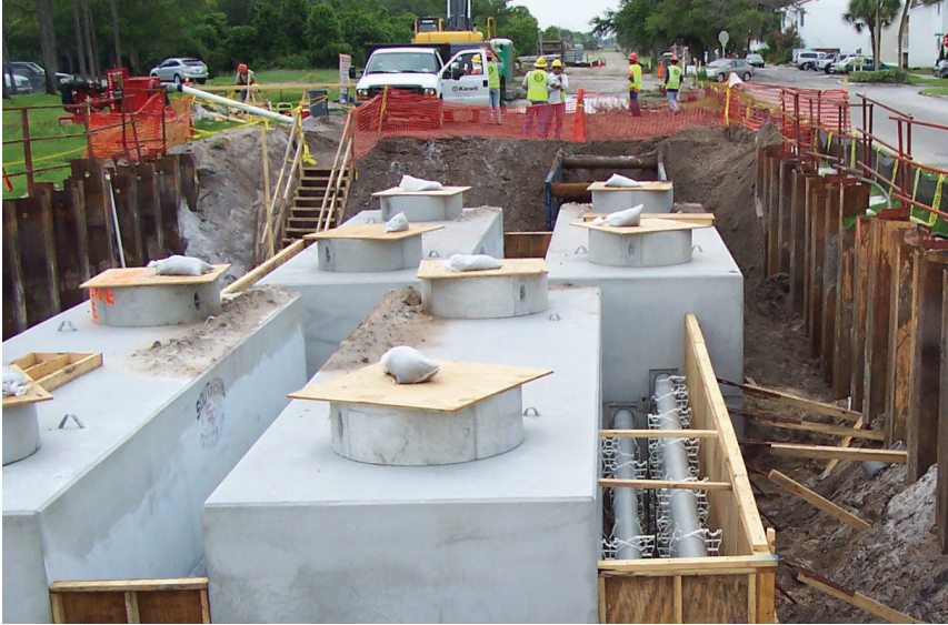
Garage-sized concrete access structures must be placed underground every 1,500 to 2,500 feet for maintenance and repair of an underground line.
