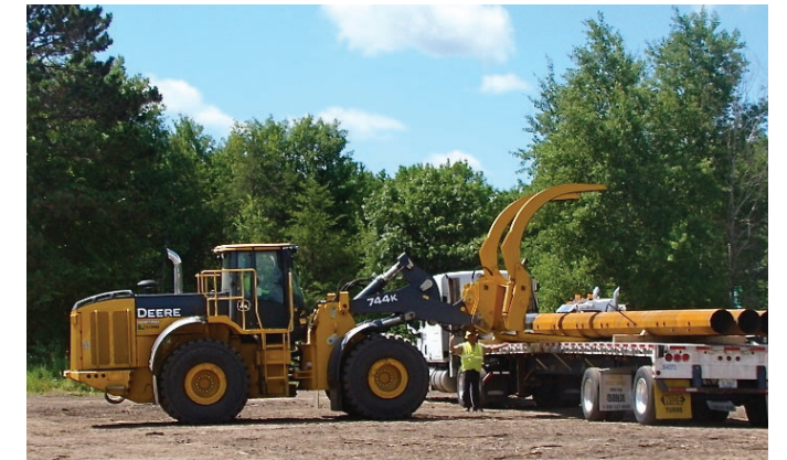
Crews unloaded transmission structures near Bena in preparation for construction to start later this summer.
