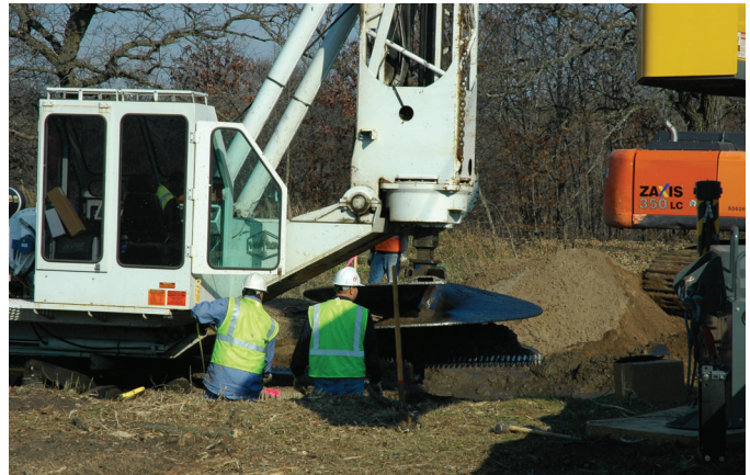
Crews operate a drill crane for the first Monticello-St. Cloud project structure foundations near Interstate 94.
